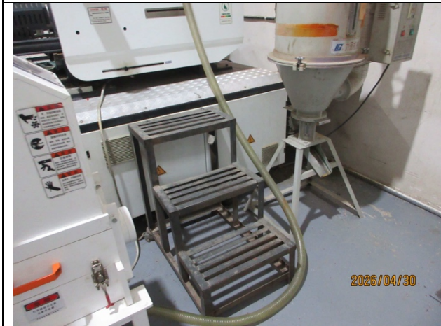
PA 7.17 No handrail for the material feeding ladder
