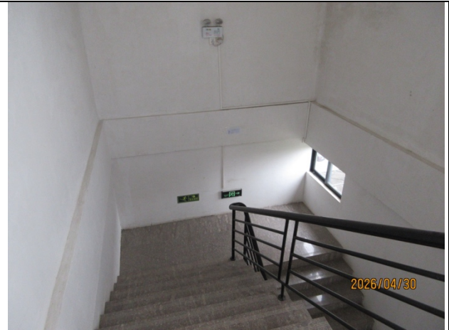
Staircase with emergency light and evacuation sign
