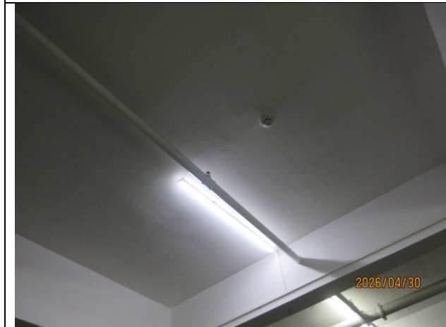
Automatic smoke detection and sprinkler system
