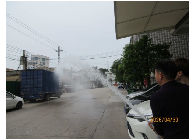
Fire hydrant testing
