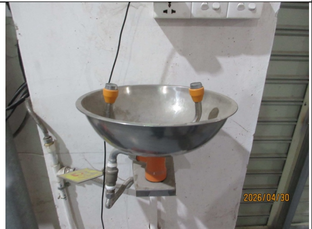
Eye wash station
