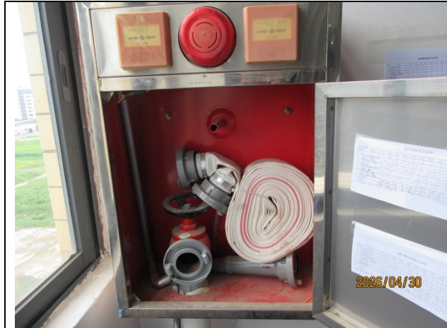
Fire hydrant and fire alarm
